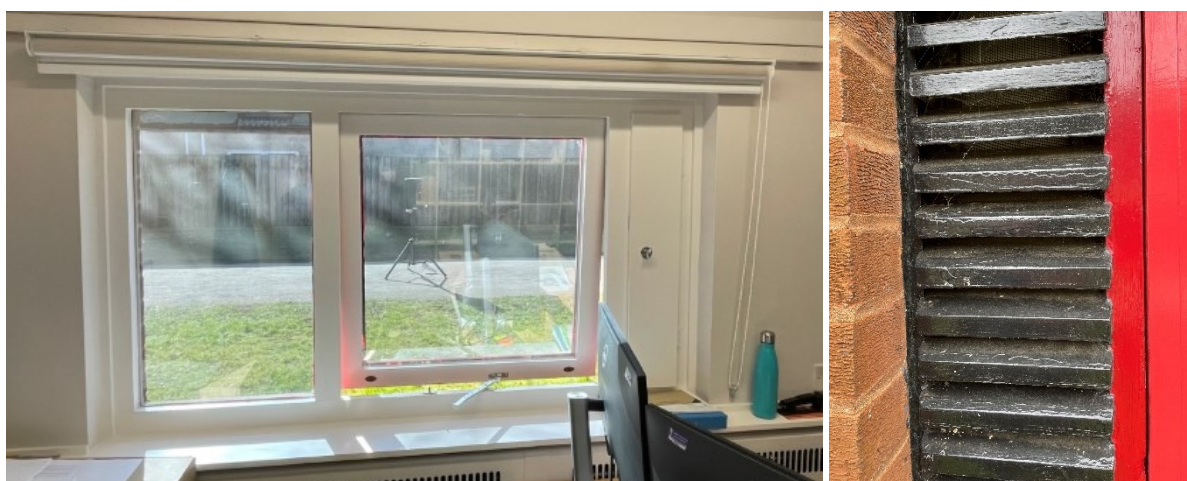
Figure 6.7: Office Window Partially Open with Ventilation Louvre Shown Closed – View of Louvre From Outside. Note: There was no Obstruction to Open Ventilation Louvres in the Study Room
