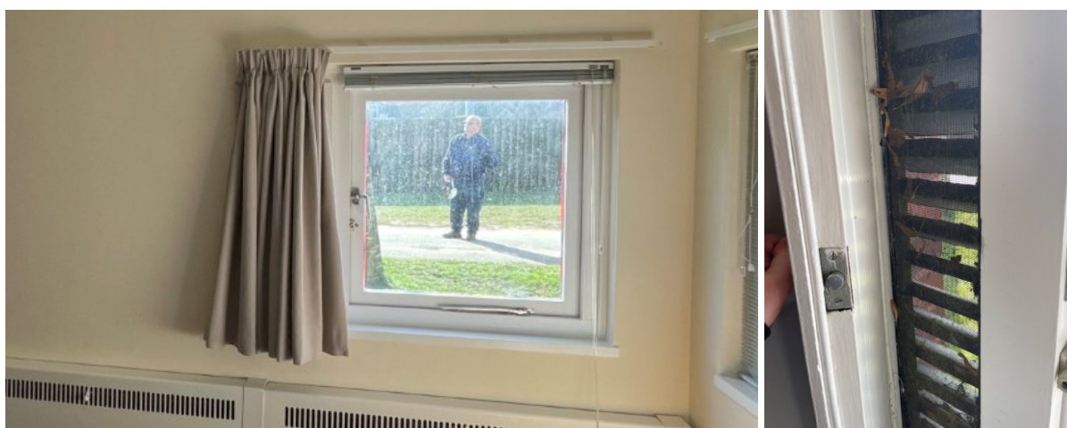
Figure 6.8: Apartment 4a Bedroom Window With Louvre Behind Curtain – View to Right of Restricted Opening for Louvre
