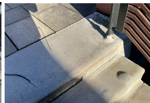
Cracked and blistered asphalt covering
