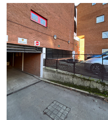
Organic and surface staining to fair faced concrete
