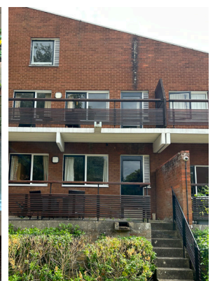
Staining to brickwork below roof trim joints
