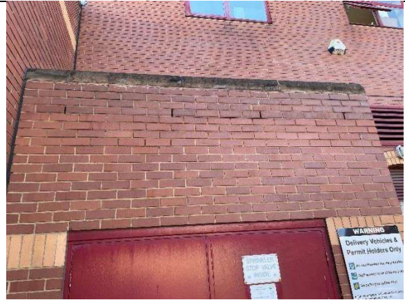
Photograph 16: Morrisons goods entrance and cracks within mortar
