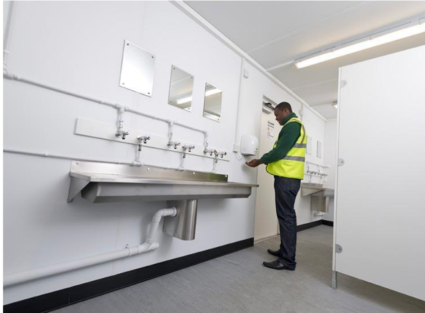
Figure 4: Typical washroom / toilet facilities
