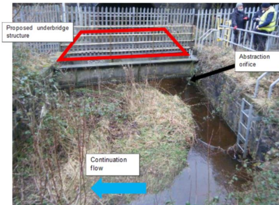
Fig. 2 - Brunclough feeder structure (abstraction orifice and continuation weir)
