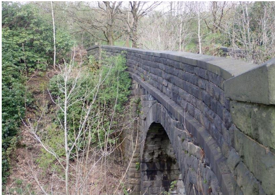
Insert 1-1 View north across the west elevation of Wright's Overbridge (MVL3/23) showing parapet out of plumb
