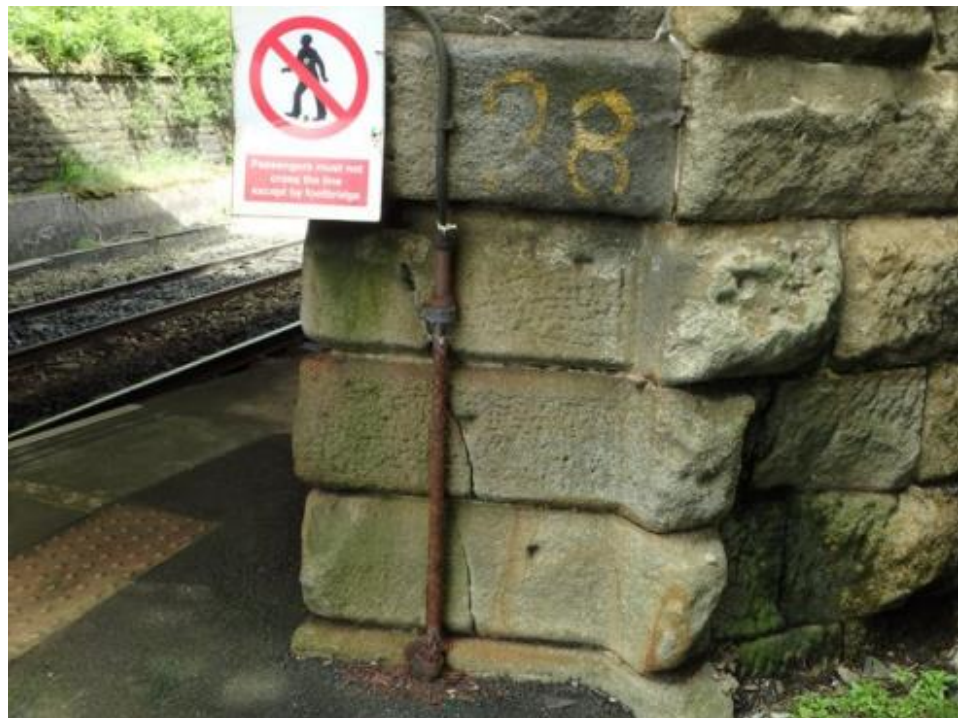
Insert 1-4 Standing fractures to the bridge abutments.
