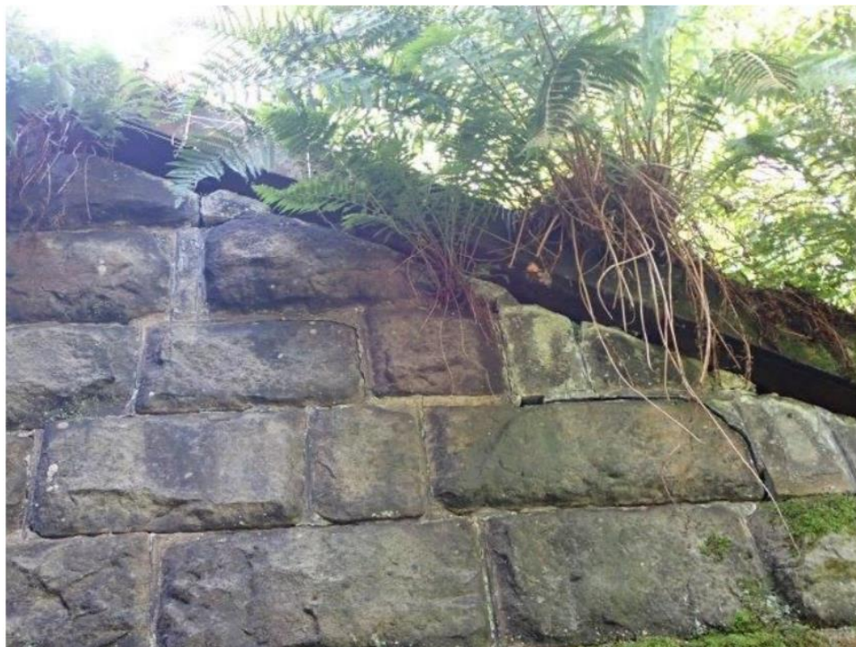
Insert 1-2 Wickens Underbridge (MVL3/29), loose, displaced and bulging stonework.
