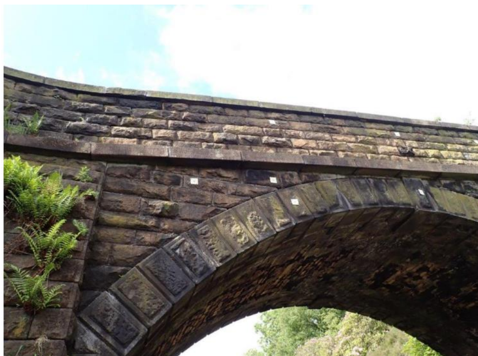
Insert 1-2 Displaced masonry and vegetation growth on Roughtown Road Overbridge MVL3/17
