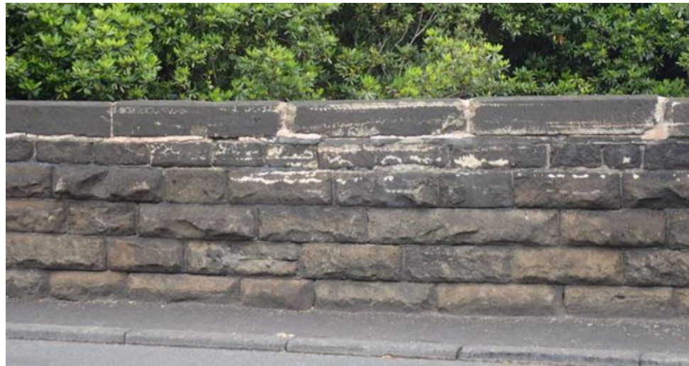
Insert 1-2 Displaced capstone on bridge parapet.
