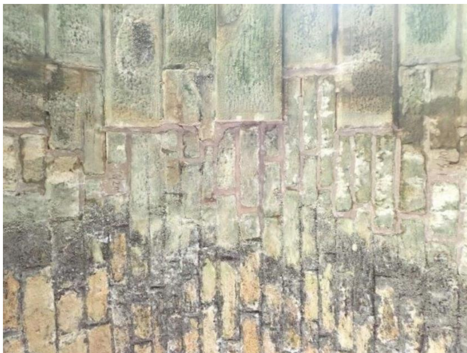
Insert 1-3 Wickens Underbridge (MVL3/29) fracture in masonry on arch.
