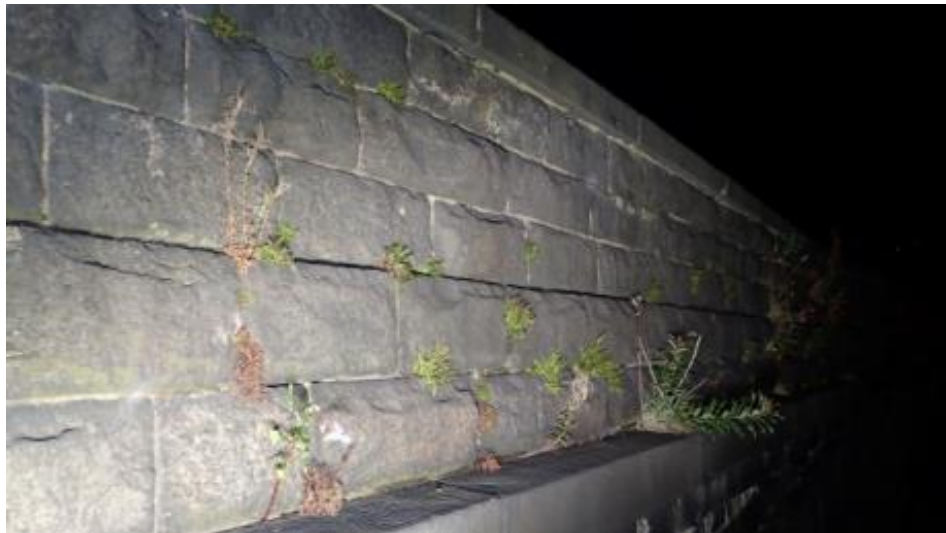
Insert 1-4 Wright's Mill Overbridge (MVL3/20), open joints and vegetation to southern parapet
