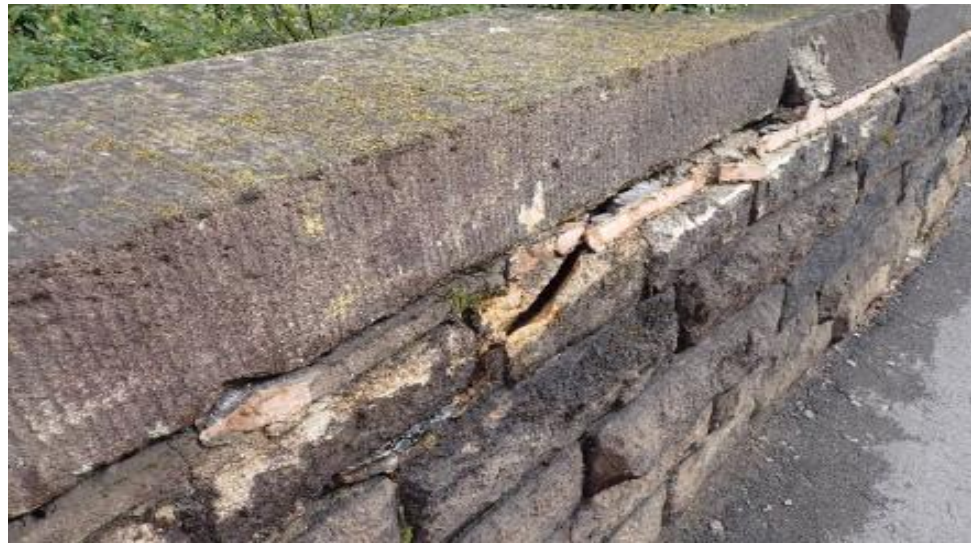
Insert 1-3 Scrape marks and displacement of coping from vehicle strikes
