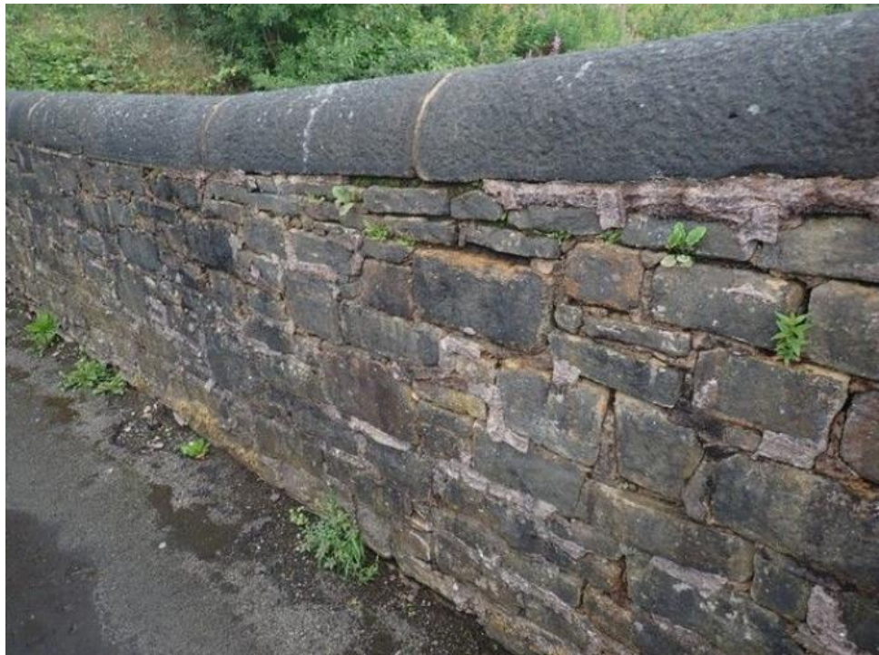
Insert 1-2 Springbank Lane Footbridge (MVL3/8), open joints and fractures to approach walls
