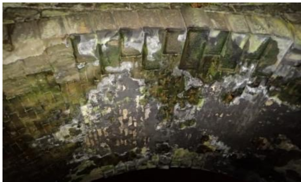
Insert 1-2 Wright's Mill Overbridge (MVL3/20), water seepage visible on arch soffit.
