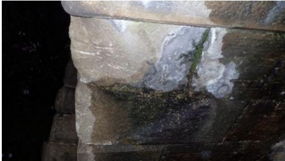
Insert 1-3 Wright's Mill Overbridge (MVL3/20), spalling on soffits.
