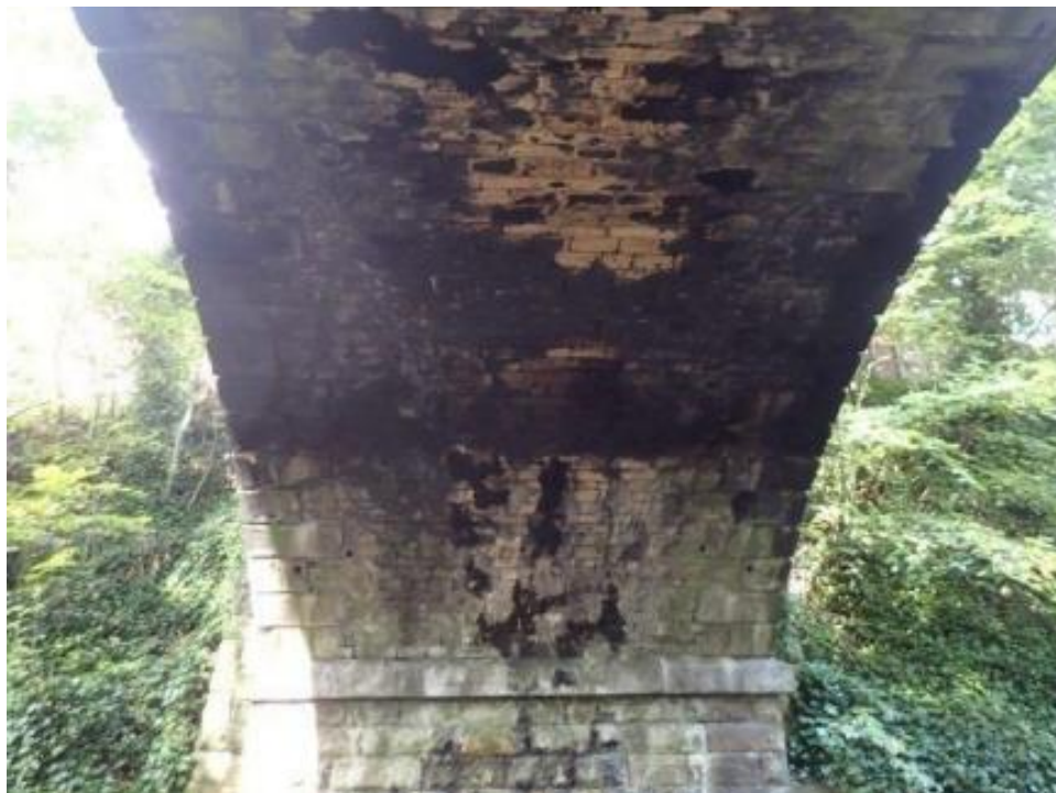
Insert 1-3 Arch soffit of Heyrod Hall Overbridge (MVL3/7) showing open joints, weathering and spalling of stonework.
