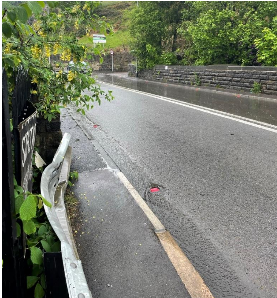
Insert 5-6 Oldham Road Bridge (MVL3/28), bridge deck and evidence of vehicle strike.
