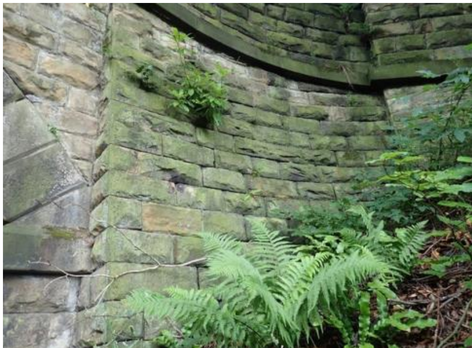
Insert 1-4 Weathering, and open joints on Heyrod Hall Overbridge (MVL3/7).
