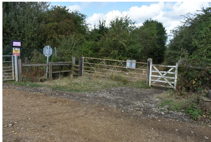
Painter Road access crossing the County Park side of the Crossing with gate and stile, the stile is clearly substandard see image below.
