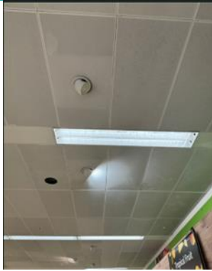
Image 65 Suspended Grid Mineral Tiles
