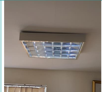
Image 124 Shopping Centre - Lighting
