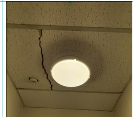
Image 64 Suspended Grid Mineral Tiles
