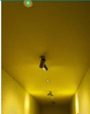
Image 121 Shopping Centre - Lighting
