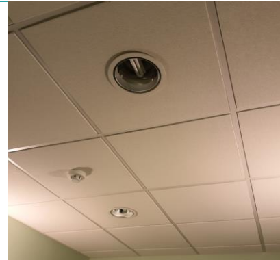
Image 119 Shopping Centre - Lighting
