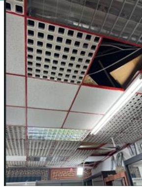
Image 67 Suspended Grid Mineral Tiles
