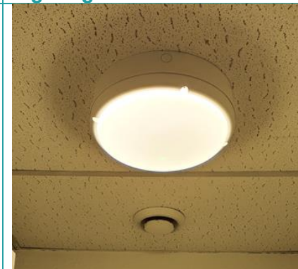
Image 112 Shopping Centre - Lighting
