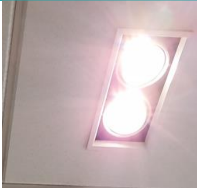
Image 113 Shopping Centre - Lighting
