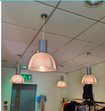
Image 117 Shopping Centre - Lighting
