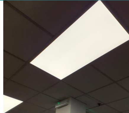
Image 123 Shopping Centre - Lighting
