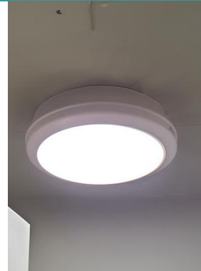
Image 115 Shopping Centre - Lighting
