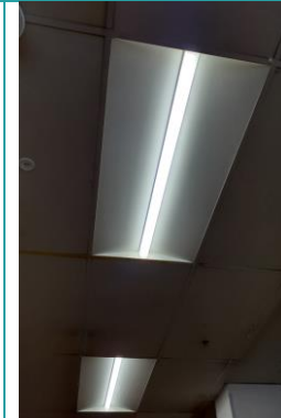
Image 116 Shopping Centre - Lighting
