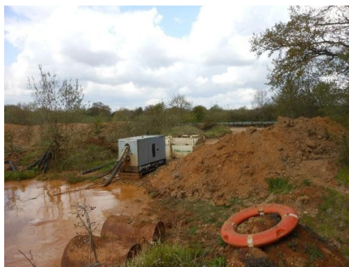
An example of active pumping
