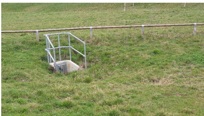
A passive swale
