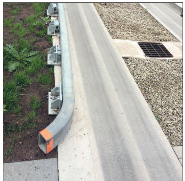
Figure 9.10 Burst through guide rail (Leigh & Ellenbrook)
