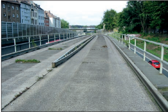
Figure 9.11 Steel guide rails mounted on concrete slab over structure, Essen (A40 route section)
