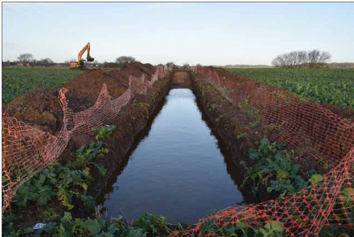
Plate 28: Trench 73 flooded, Field 7b, looking north-west
