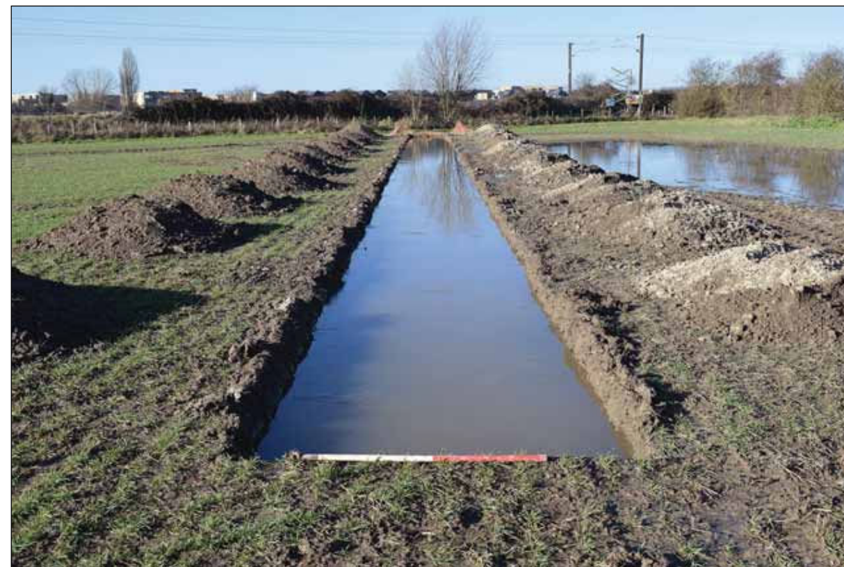
Plate 6: Trench 4 flooded, Field 2, looking north-west
